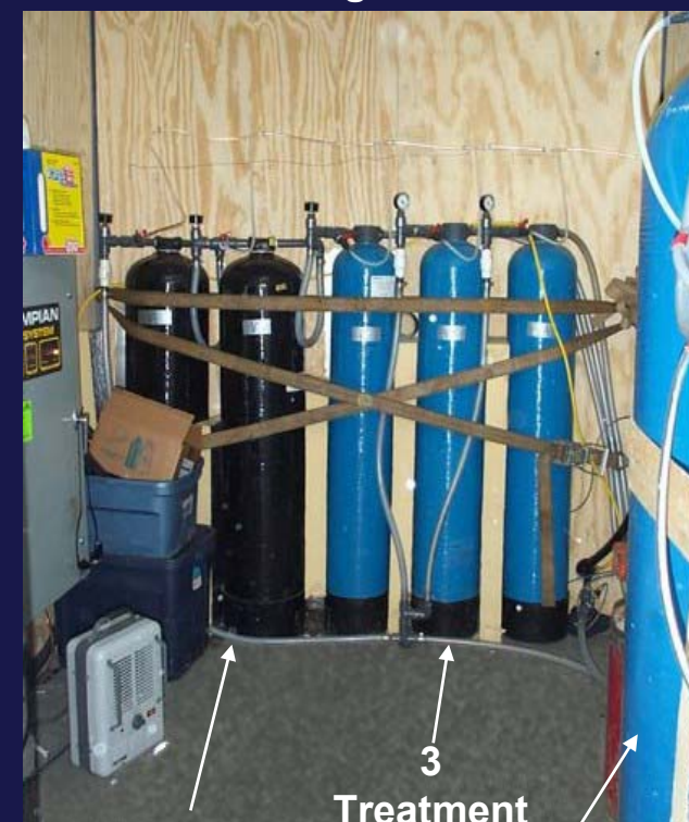
2 Polishing Vessels for Tailored GAC Unit 3 Treatment Vessels Final Polishing Vessels
