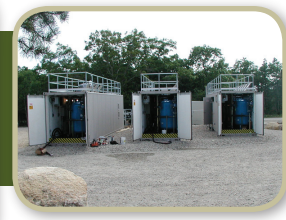
Modular groundwater treatment units
