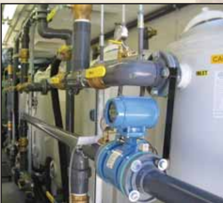
Interior of a modular treatment unit.
