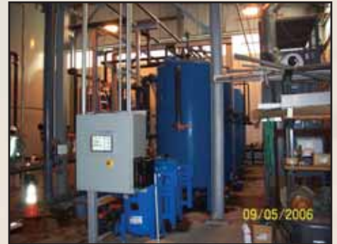
The IAGWSP's J-3 Range Plume treatment system is located in an unused corner of the IRP's FS-12 treatment facility.
