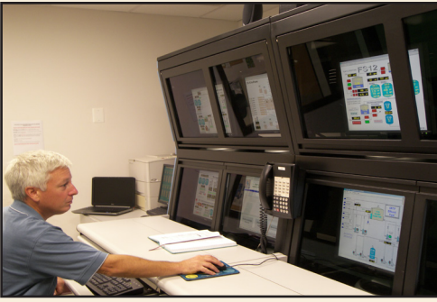
The status of AFCEC groundwater cleanup systems in the control room at AFCEC's Operations and Maintenance Facility.
