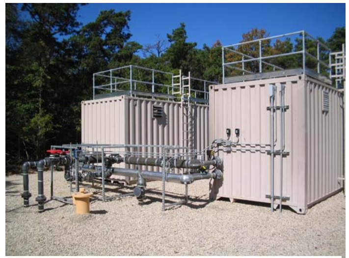
MTUs E and F at the J-2 northern plume – Installed under an interim response action in 2006
