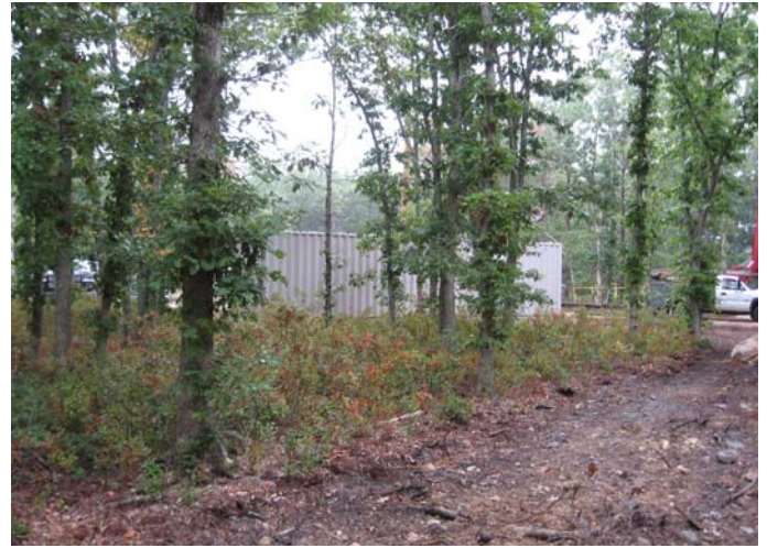
Southern J-1 Range Treatment Unit – Installed under a Rapid Response Action in October 2007
